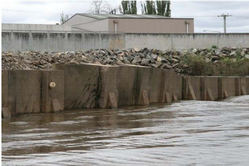
Siltation impact on Tamar River retaining wall
