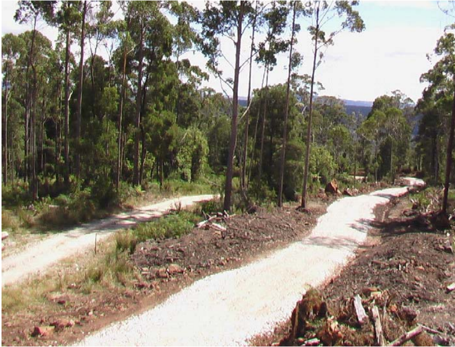
New road on the right parallel to and a few metres from the original access road.
