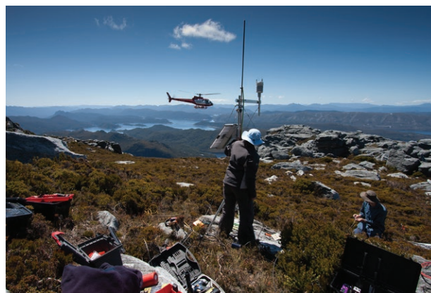
INSTALLING AN AUTOMATIC WEATHER STATION ATOP MT SPRENT AS A HELICOPTER USED TO OFFLOAD THE RESEARCHERS AND EQUIPMENT, FLIES PAST, WITH LAKE PEDDER VISIBLE IN THE DISTANCE - Photo: N Fitzgerald
